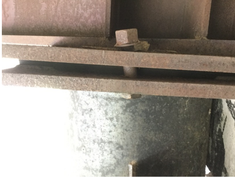
Upstream left bank bearing bolt
