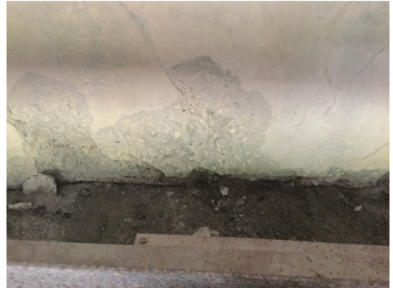
Right bank ballast wall damage
