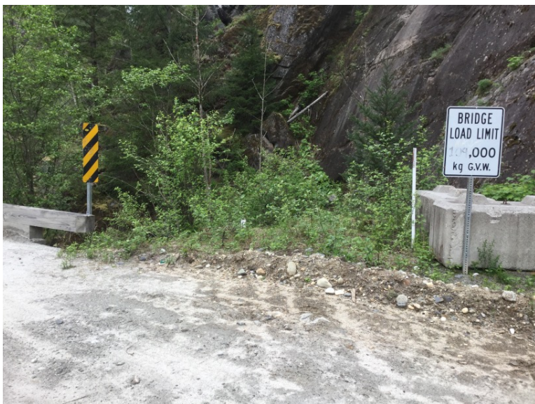
Missing upstream left approach barrier
