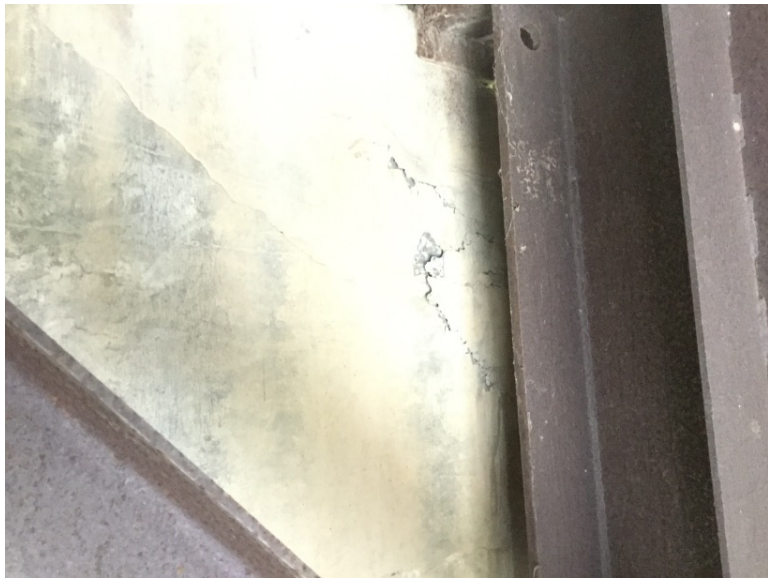
Right bank ballast wall damage
